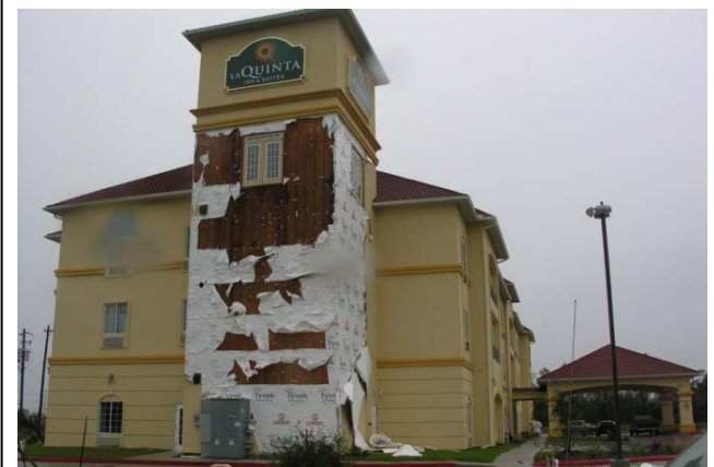
Source – Institute for Business & Home Safety Wind damage to lightweight exterior wall covering.
