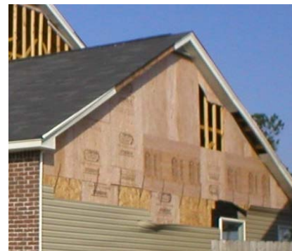
Source – Portland Cement Association – photo by Steve Skalko Damage to siding and sheathing as a result of high winds
