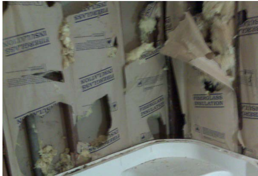
Source: Image provided with permission from Alternative Building Services: www.altbuildingservices.com .
