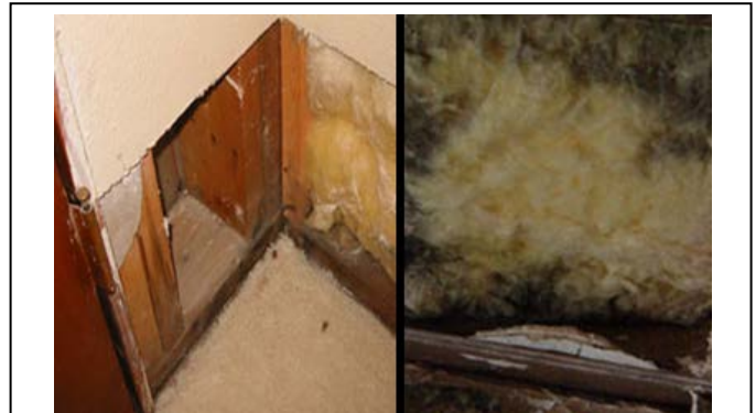
Source: FEMA - contributed by John Martyny
